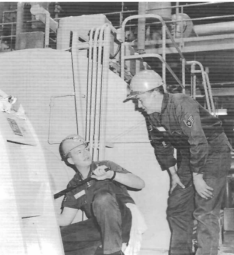
◀ Staff sergeant and airman working on one of the four diesel generators in a Titan I powerhouse.
